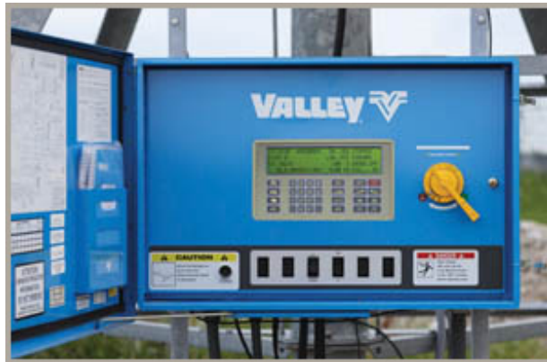
Auto Pilot Control Panel
