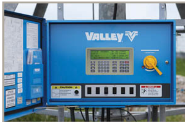
Auto Pilot Control Panel
