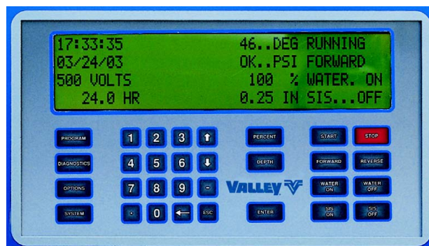
Valley Pro2 Control Panel
